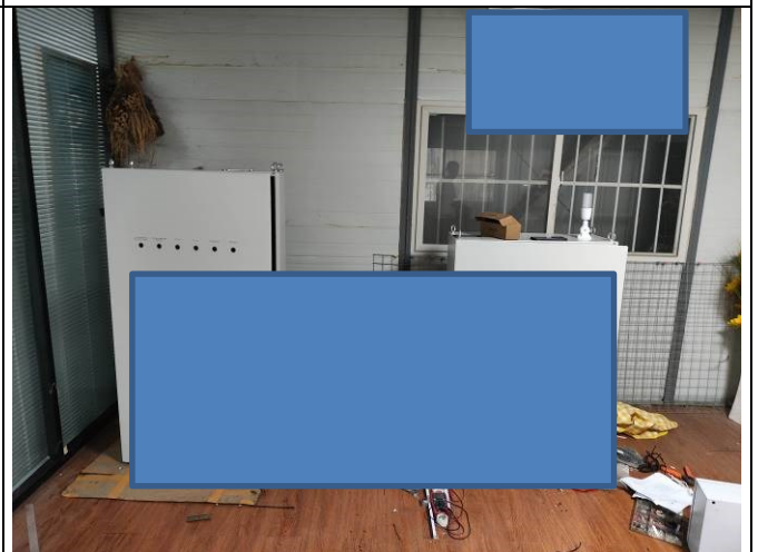
Electricity installation as per drawing
